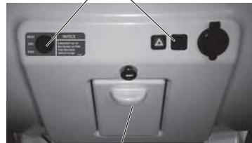
Electrical Access Panel (Fuses/Main Disconnect Switch)
